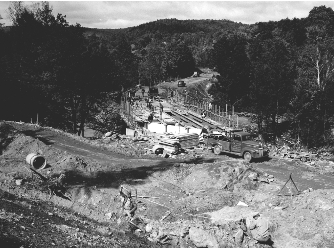
Construction of the bridge over the Ompompanoosuc River on Route 132, part of the Union Village Dam project, ca. 1947.
