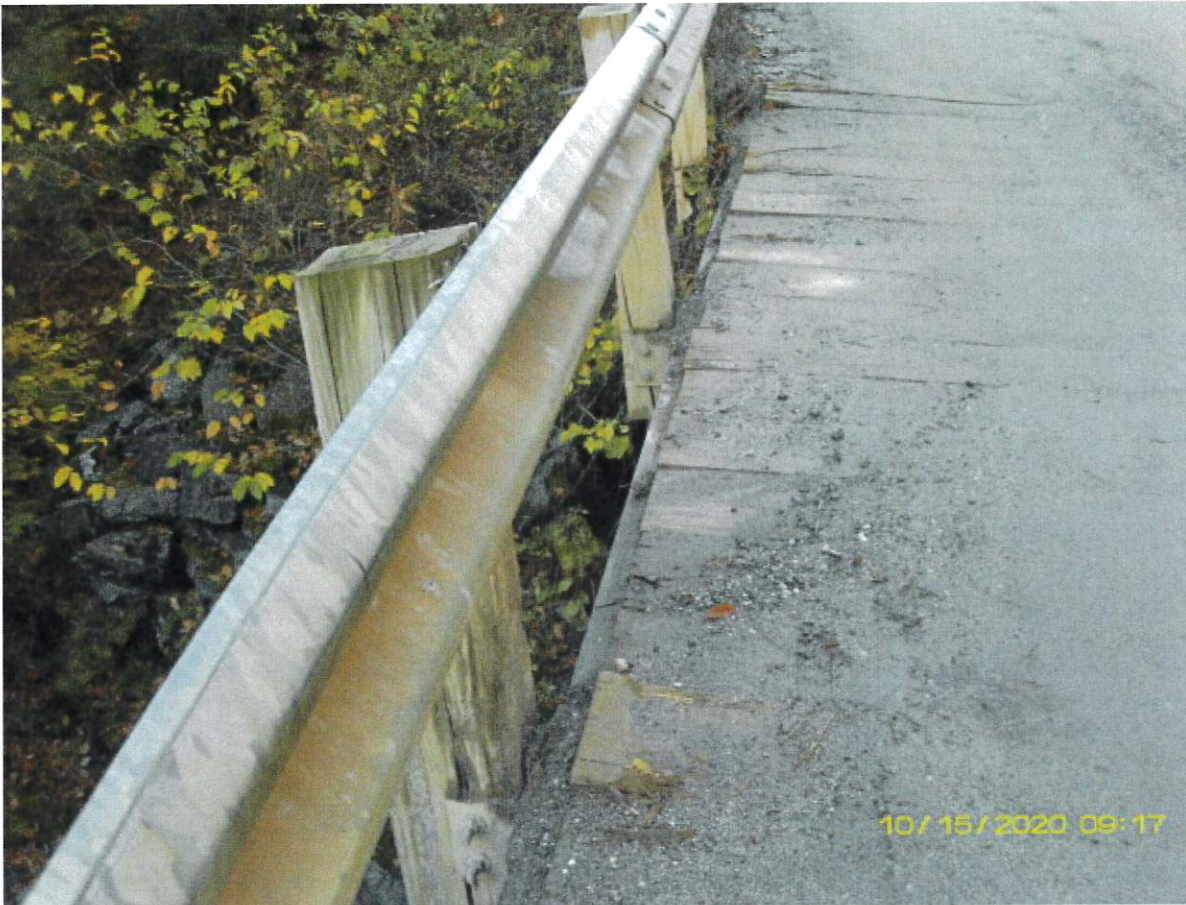
Stowell Road Bridge – Failing Wood Bridge Rail Posts
