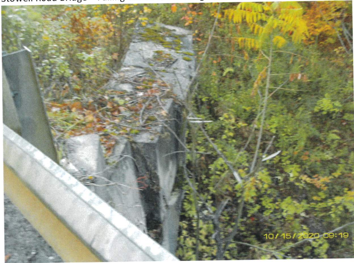
Stowell Road Bridge – Failing Waste Block Wing Wall
